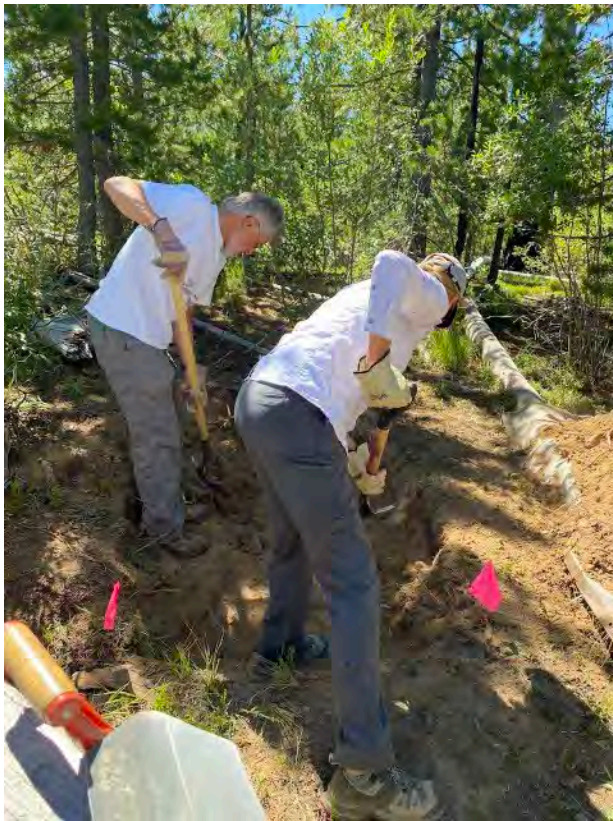
Those with strong backs helped to dig a trench in search of the fault line.
