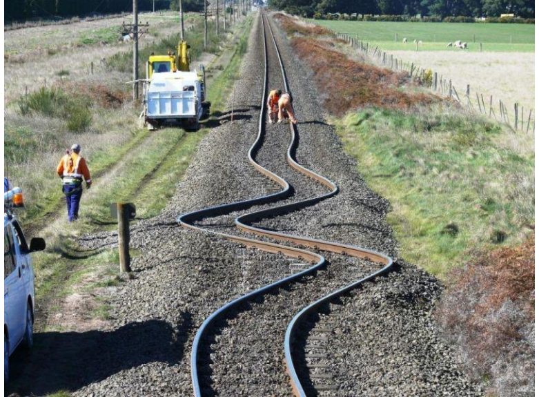
Typical track deformation due to ground surface motion in an earthquake.
